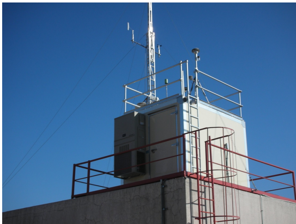
Figure 3-4. Photo of AJM Ambient Site Shelter on Roof of Hospital
