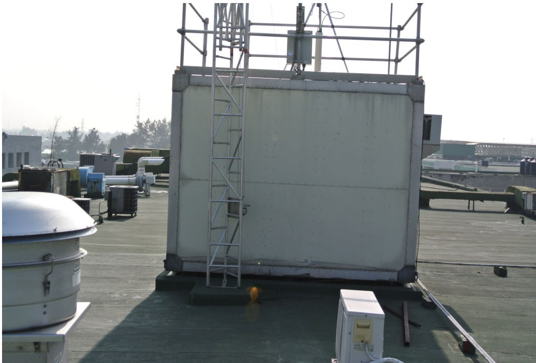
Figure 3-9. Rear View of the UIZ Ekto Shelter
