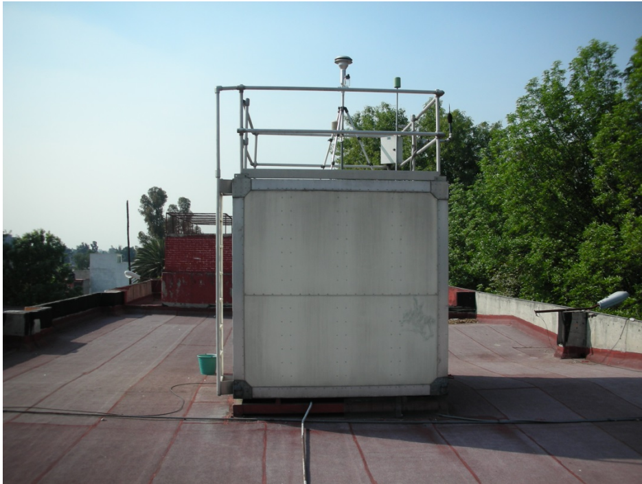
Figure 3-12. Side View of Ekto Shelter at SJA Site, Looking West
